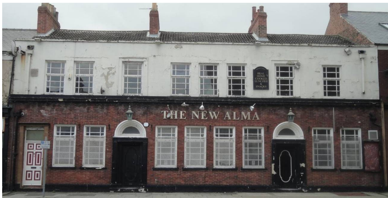
Fig 46. The New Alma, Whitby Street, showing failing paint and render and dampness.
