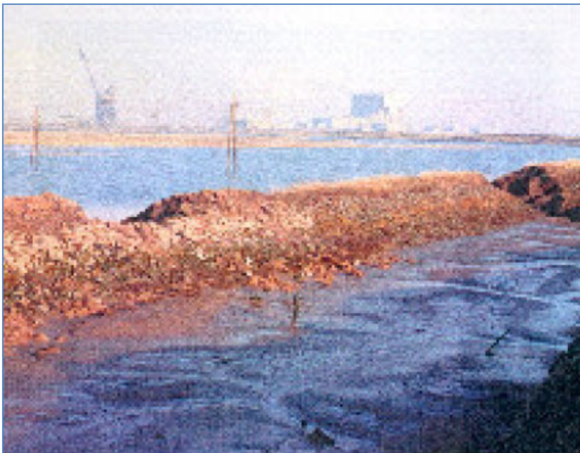
Figure 4 - Breach of Greatham North embankment in 1978
