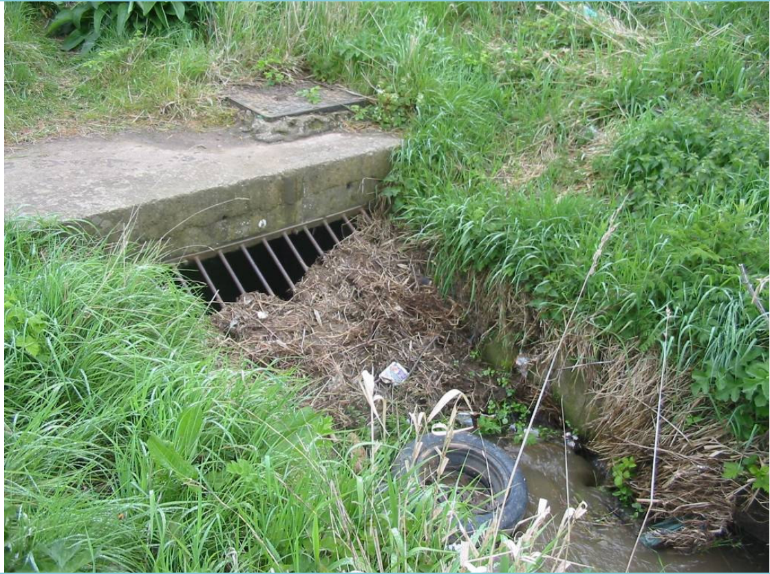
Figure 4-2: Middle Warren Watercourse Culvert Inlet Trash Screen
