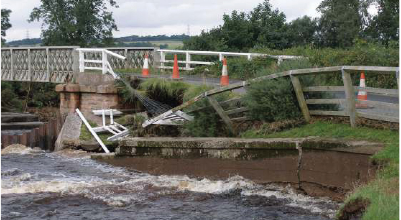
Erosion of southern bridge abutment at Ingram during flood in September 2008
