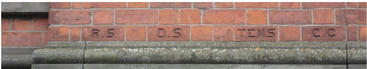
Fig 30. Initials of patrons incised into the brickwork at Wesley Methodist Church.
