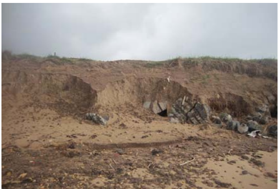
Plate 3: Failure/erosion of emergency capping works (MARCH 2012)
