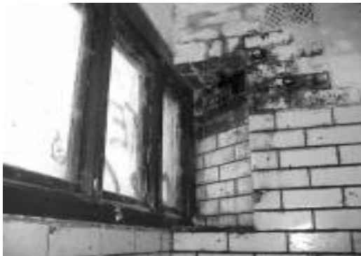
An illustration of the deteriorating condition of the Thorpe Street facility.
