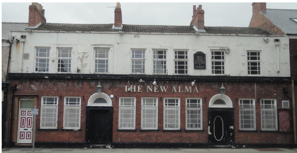
Fig 44. The New Alma, Whitby Street, showing failing paint and render and dampness.
