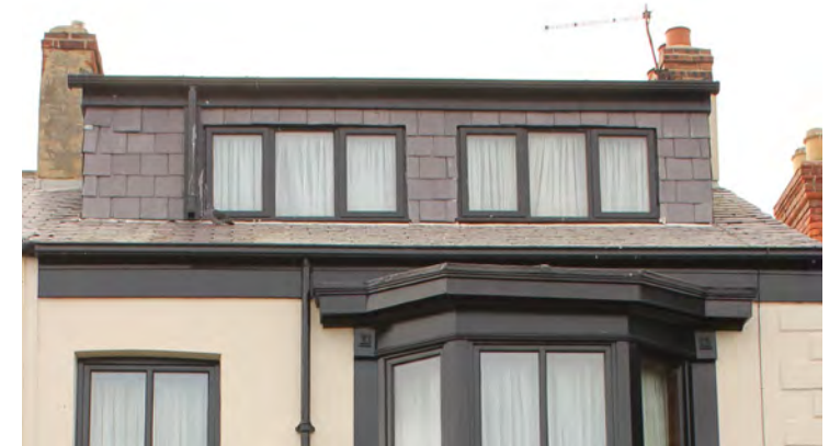
Inappropriate dormer on an historic building
