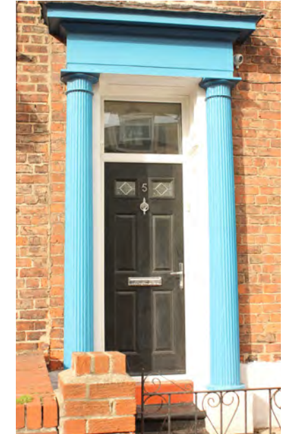
A modern composite door incorporating glazing and modern chrome fittings is not appropriate.
