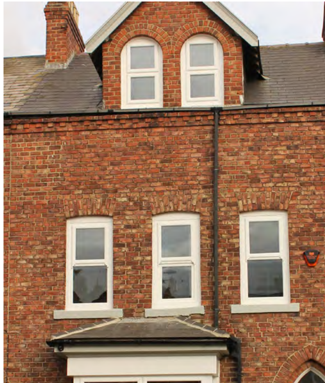
An example of inappropriate uPVC windows; the frames are too heavy, their standard shape fails to respond to the arched window openings and make a poor attempt to imitate sashes.
