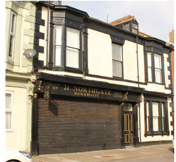
Solid roller shutters on Northgate are intrusive on this tradition shop front
