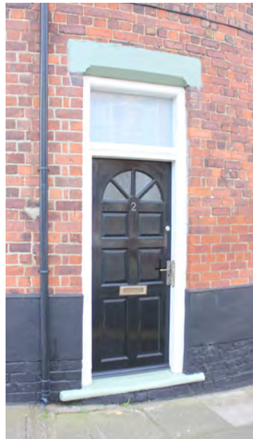
Although timber, this style of door is a modern reinterpretation which is not appropriate on historic buildings.
