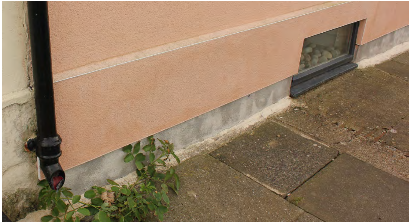
This modern render is raised above the finish on the adjacent building and has a distinctive plastic edging strip. If utilising a modern impermeable material, it may be causing more harm than good on this historic building.
