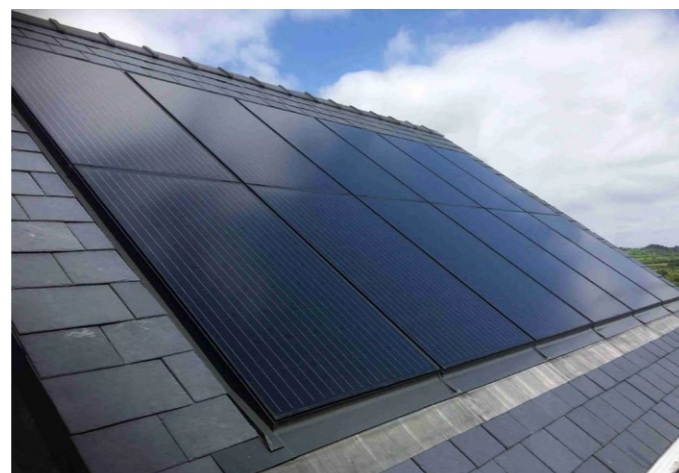
Solar panels on roof
