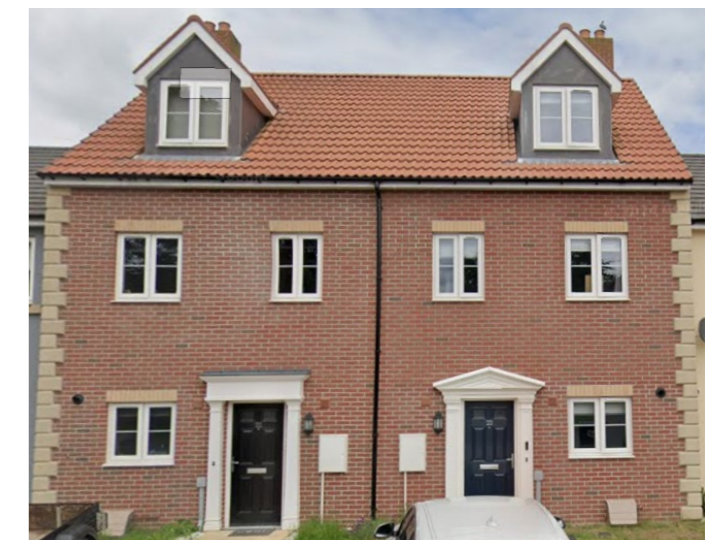
Meter box impacting on elevation
